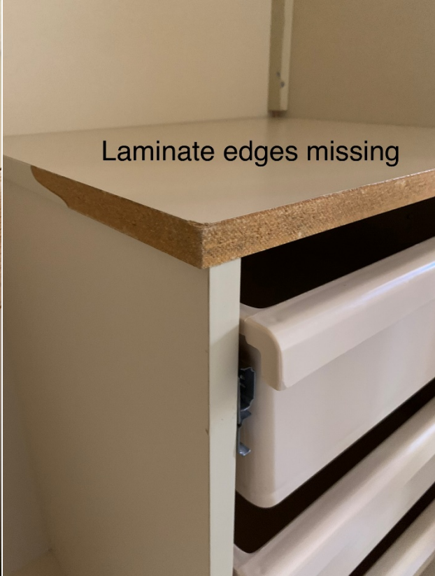
Particle wood expansion & laminate peeling
